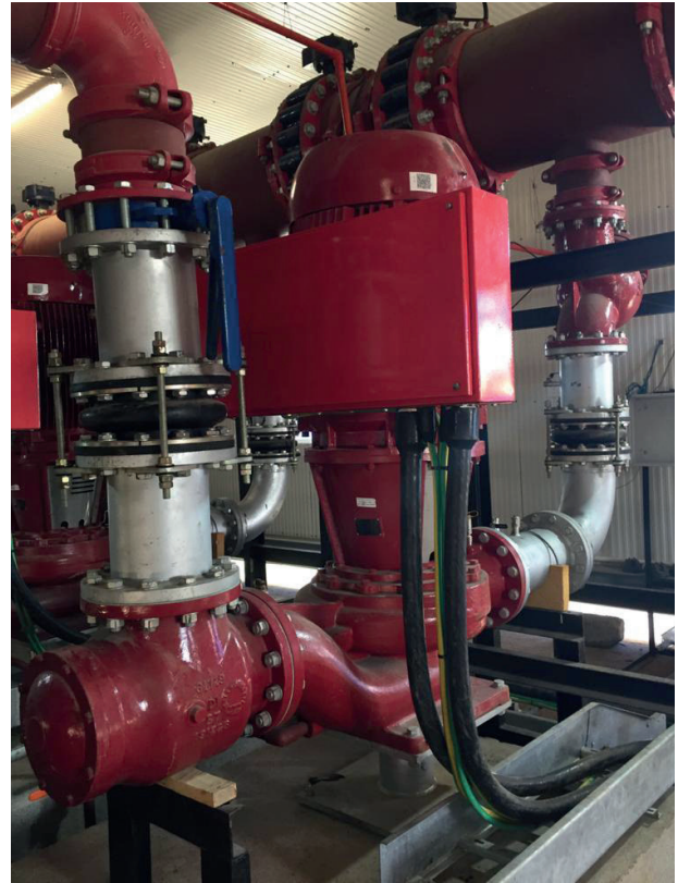
Series e-80SCXL installation at a data center in Dubai.
